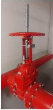
DIESEL SUCTION VALVE
