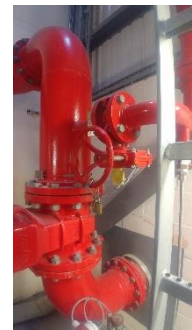
PUMP HOUSE VALVE
