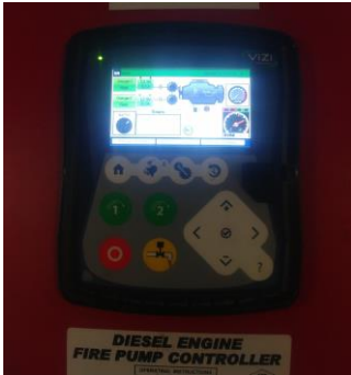
DIESEL CONTROL PANEL
