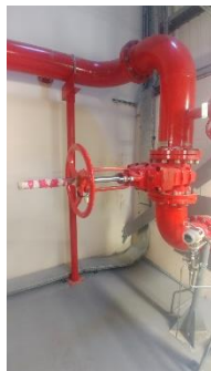
UNDERGROUND PIPE VALVE
