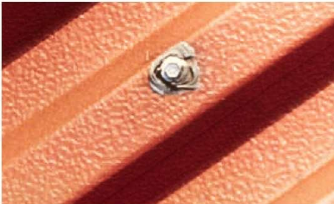
Damaged fastener on roof cladding.
