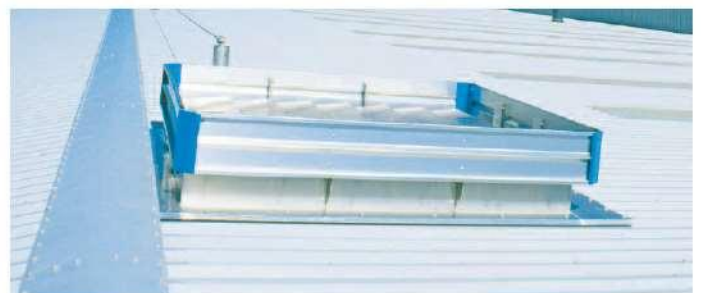
A penetration in roof cladding.
