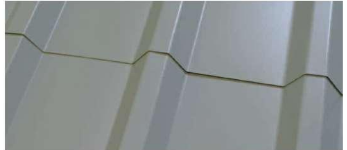
Cut edge on roof cladding.
