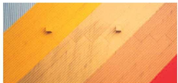
Dirt build up on cladding.
