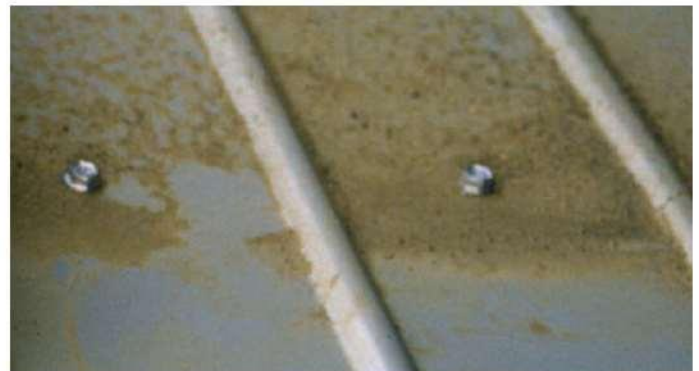
Mould growth on pre-finished steel cladding.
